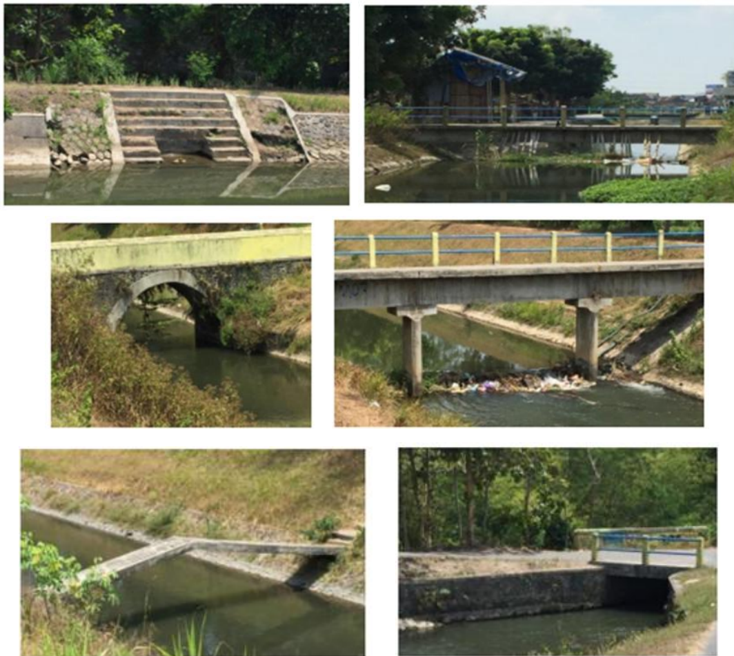
Figure 2. The Deteriorated Condition of Selokan Mataram, Including Leakage, Bridge Erosion, Waste Accumulation, Bridges Positioned Too Close to the Water Surface, and Bridge Designs Unsuitable for Tourism Activities.
